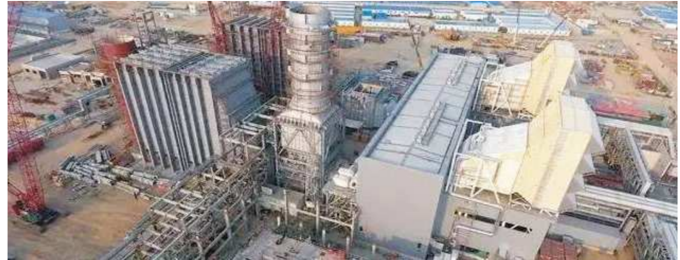
Balloki 1180MW Combined Cycle Power Station in Pakistan
